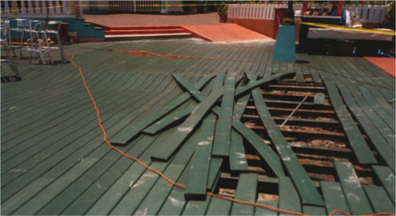
Figure 4: Buckling of a wood thermoplastic composite in the Bahamas.
